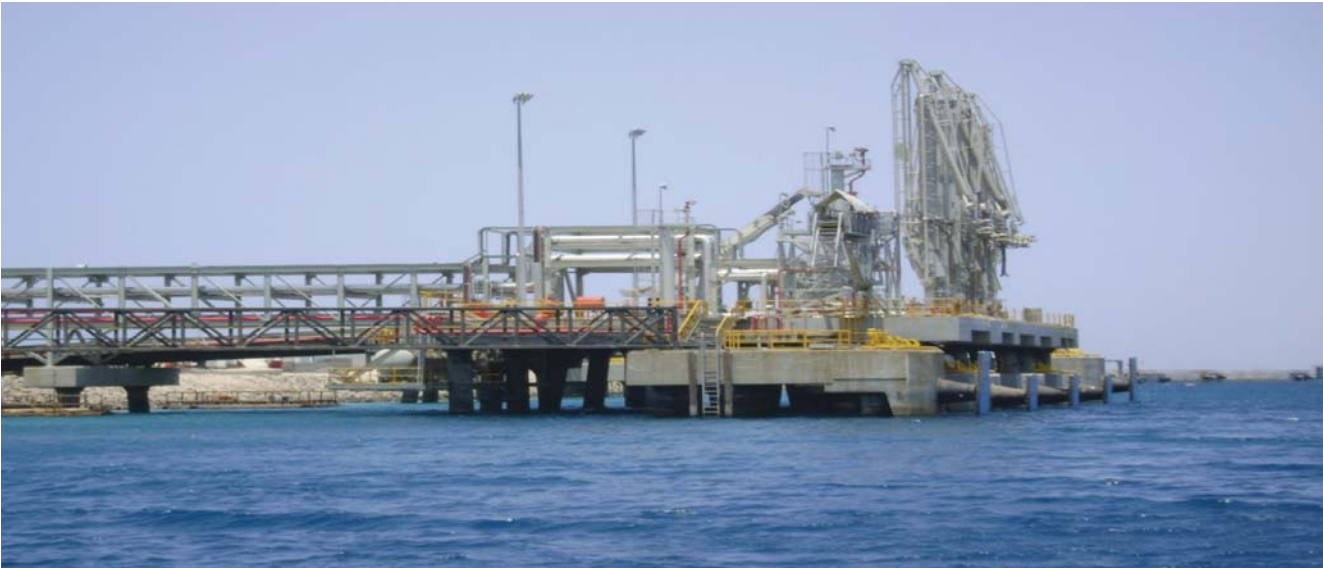
Loading Arm of LNG Terminal at one of the Middle East Country
