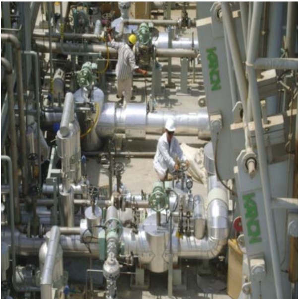
Actual Installation with Heavy Insulation
